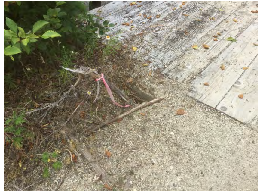
Failing fill at right bank
